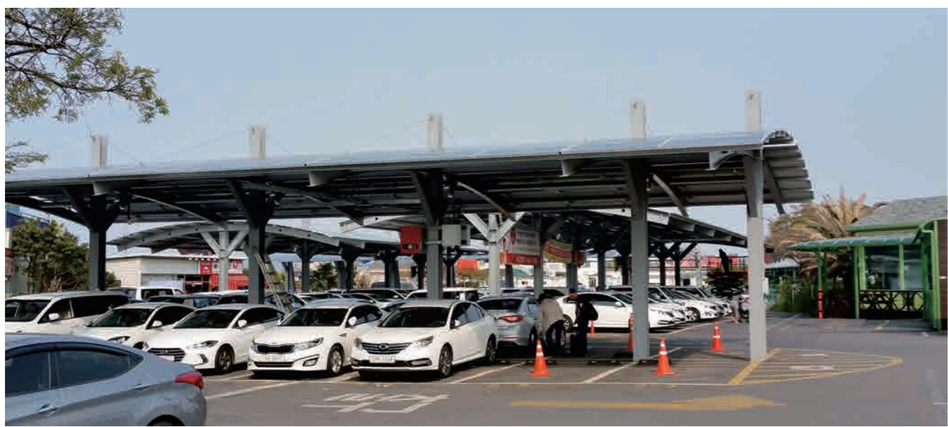
185kW, PV Carport, South Korea
