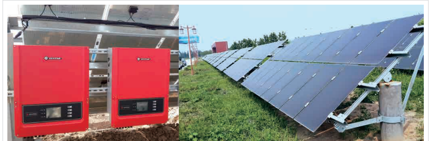
250kW, Shangdong, China
