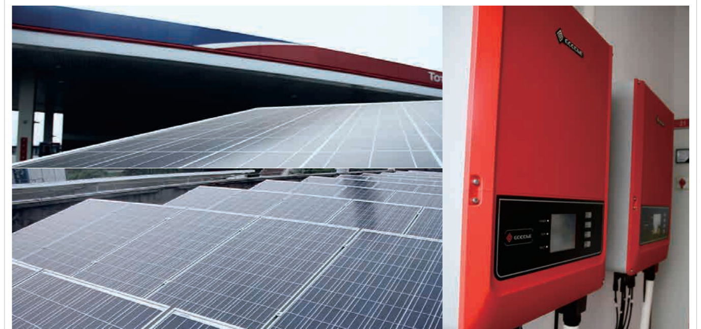
30kW, Petrol station
