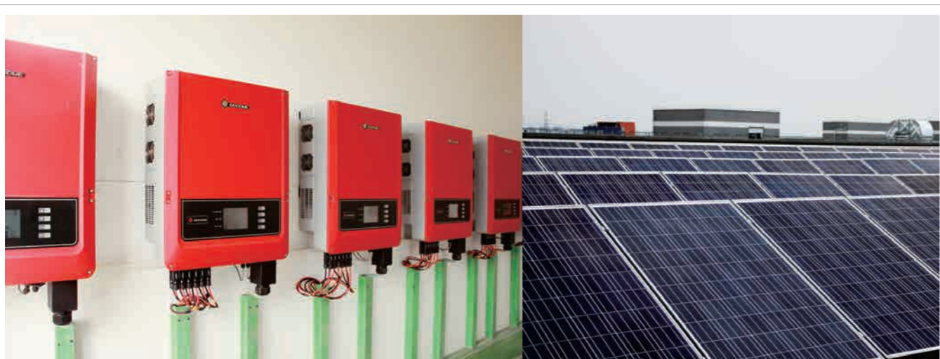
500kW, Shanghai, China
