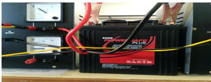
Fig 5. Exide Power plus, Lead-acid battery
